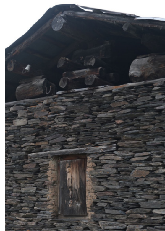
Figure 43 - Roof of the tower rested on the crown support "qorbegela". (My photo)
